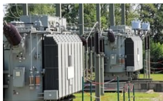
Electrical Power Distribution
